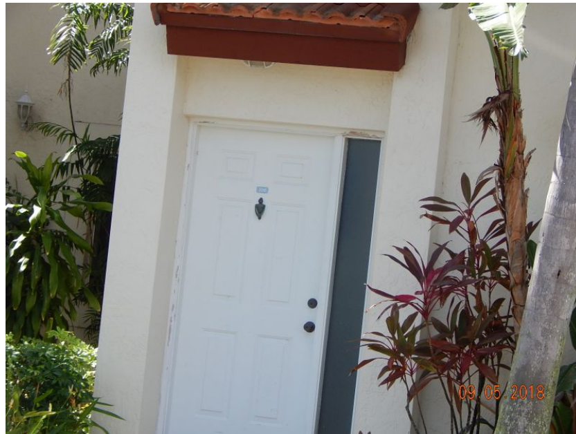
Unprotected Solid Entry Door
