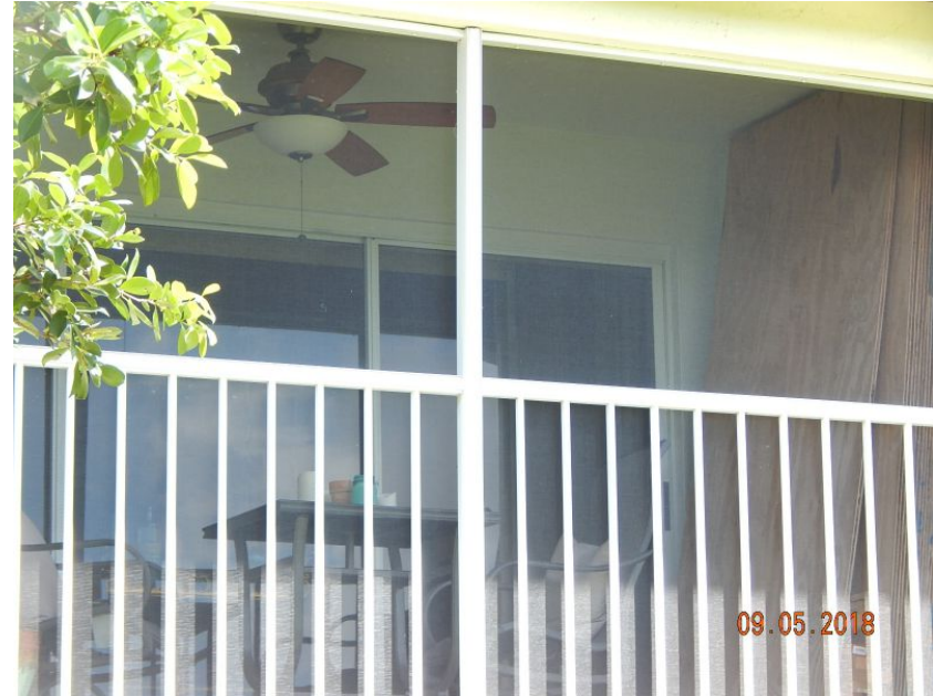
Unprotected Glazed Entry Door
